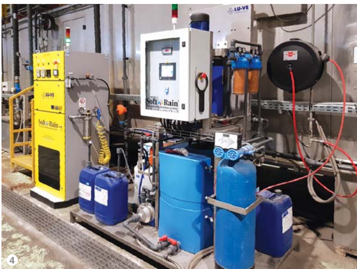
Figure 4: A detail of the Soft Rain system.
