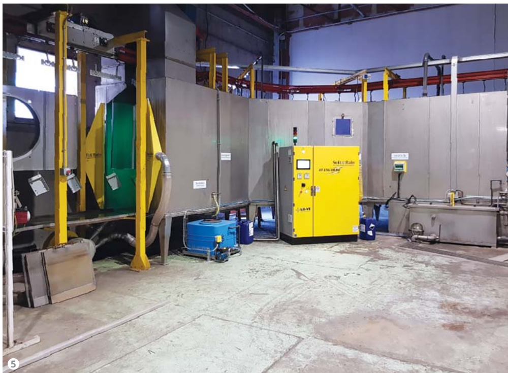
Figure 5: The Soft Rain Avantgarde system was integrated into the tunnel as an innovative technology for the mixing of the nanotechnology solution.
